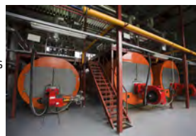
Boilers & Process Heat
