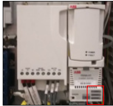
Figure 4-19: VFD Lights Turned Off
