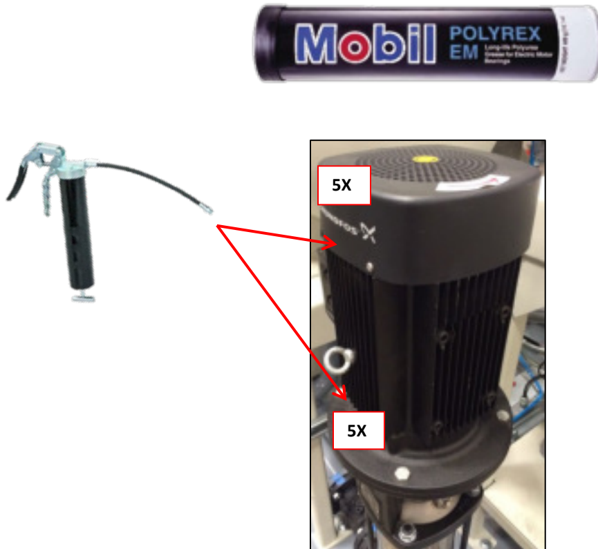
Figure 4-1: Grease Pump Motor Bearings
