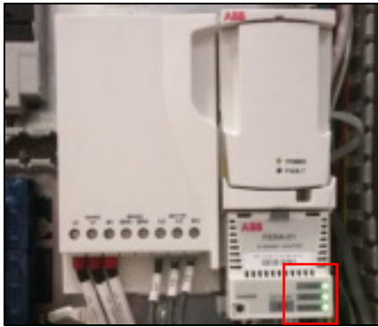
Figure 4-18: VFD Lights Still Active
