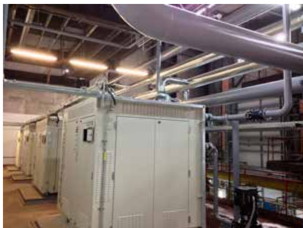
Figure 2. Electra Therm installed ten Power+ Generator 4400s at a district heating plant in Slovakia.
