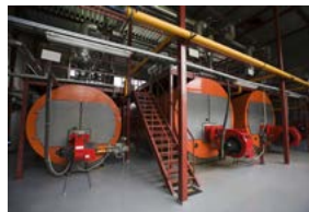
Boilers & Process Heat
