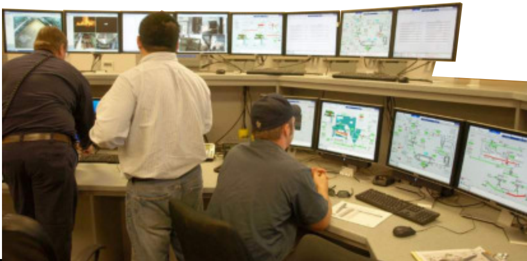
Operator control room for a biomass system
