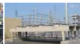
Transformer station New Orleans / USA
