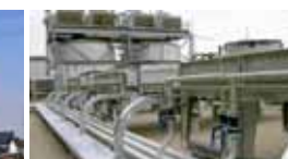
Transformer station Winnipeg / Canada
